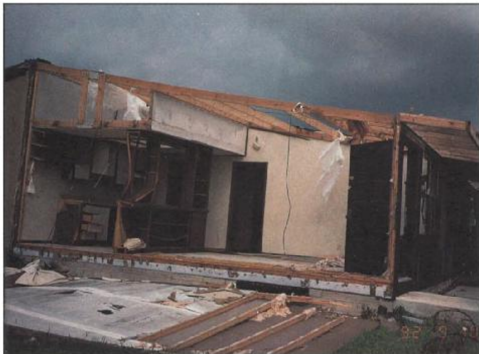
FIGURE 19. Modular home. End wall of end unit separated from unit; withdrawal of nails along eave line and roof sheathing failure were also observed.
